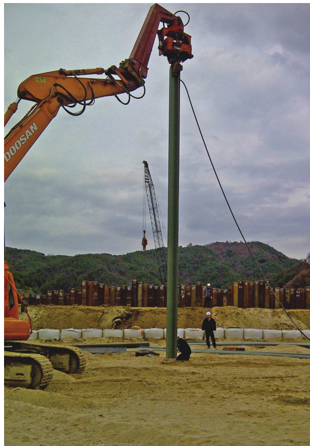
South Korea. GW-580 / 7,0 Flood banks protection.
