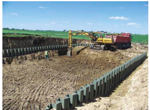
Kowal, Poland. GW-580 / 7,0 Retention tank by the A1 motorway.
